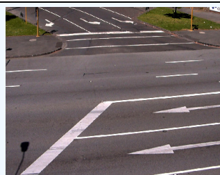
Too much bitumen?
