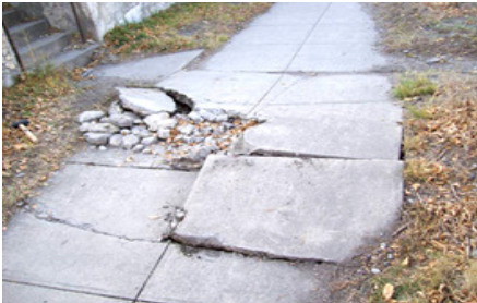
We guess that pedestrians would see this hazard, even though it's not painted yellow.
